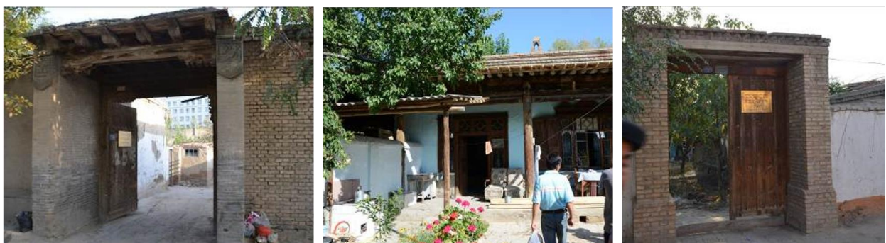
Fig.6 The building is urgent to rescue and repair
