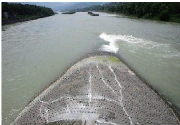
Fig.6 slight crevices on the Fish Mouth Levee 7
