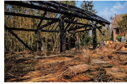
Fig.4 Damaged thatched house 2)
