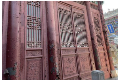
Fig. 3 Paint peeling off
