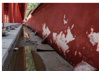
Fig.5 paint peeling off 5)
