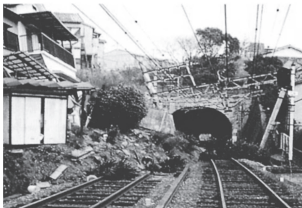
Fig.6. Collapsed tunnel near Nagata Station (Kobe Electric Railway)
