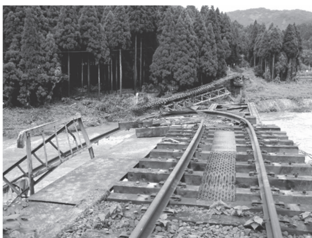
Fig.7. Broken bridge (Asuwa Dai-3 Bridge)
