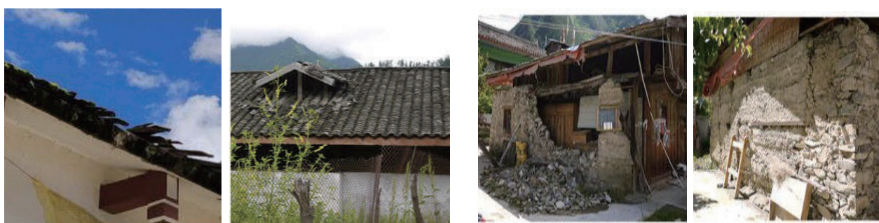
Fig. 15 Comparison of Roof Damage Repair
