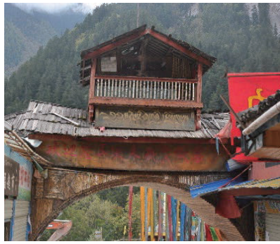
Fig. 7 Ridge of the Roof Broken
