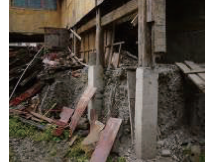
Fig. 11 Most of Wall Collapsed
