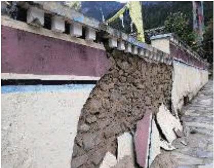
Fig. 9 The Wall Materials Fell
