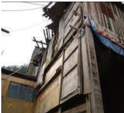
Fig. 13 Few Structures Damaged
