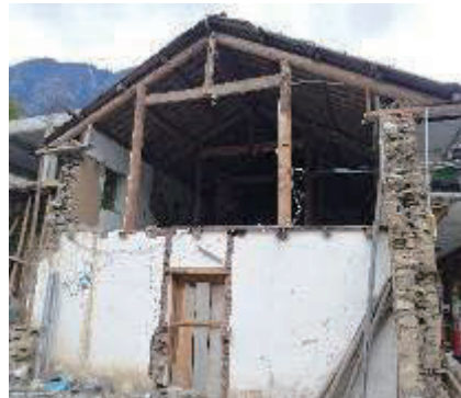
Fig. 14 Most Structures Damaged
