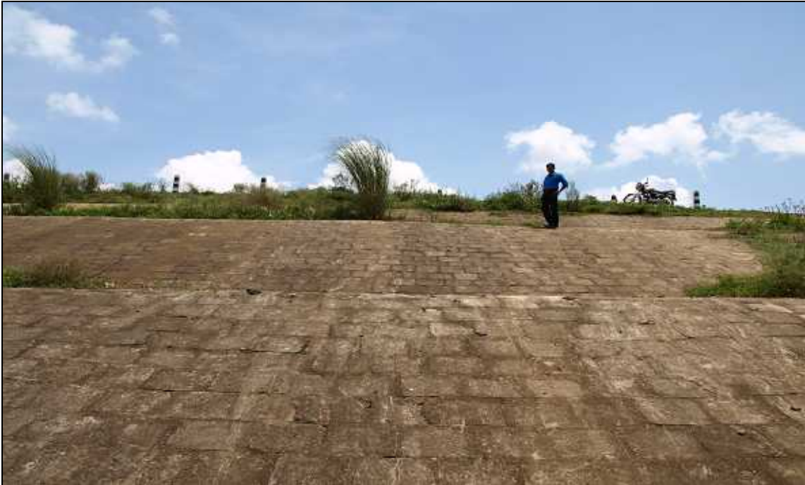
The stone cobbled embankment of Ajoy near Ilambazaar. When it comes to protection from floods, the urban centers have the priority.
