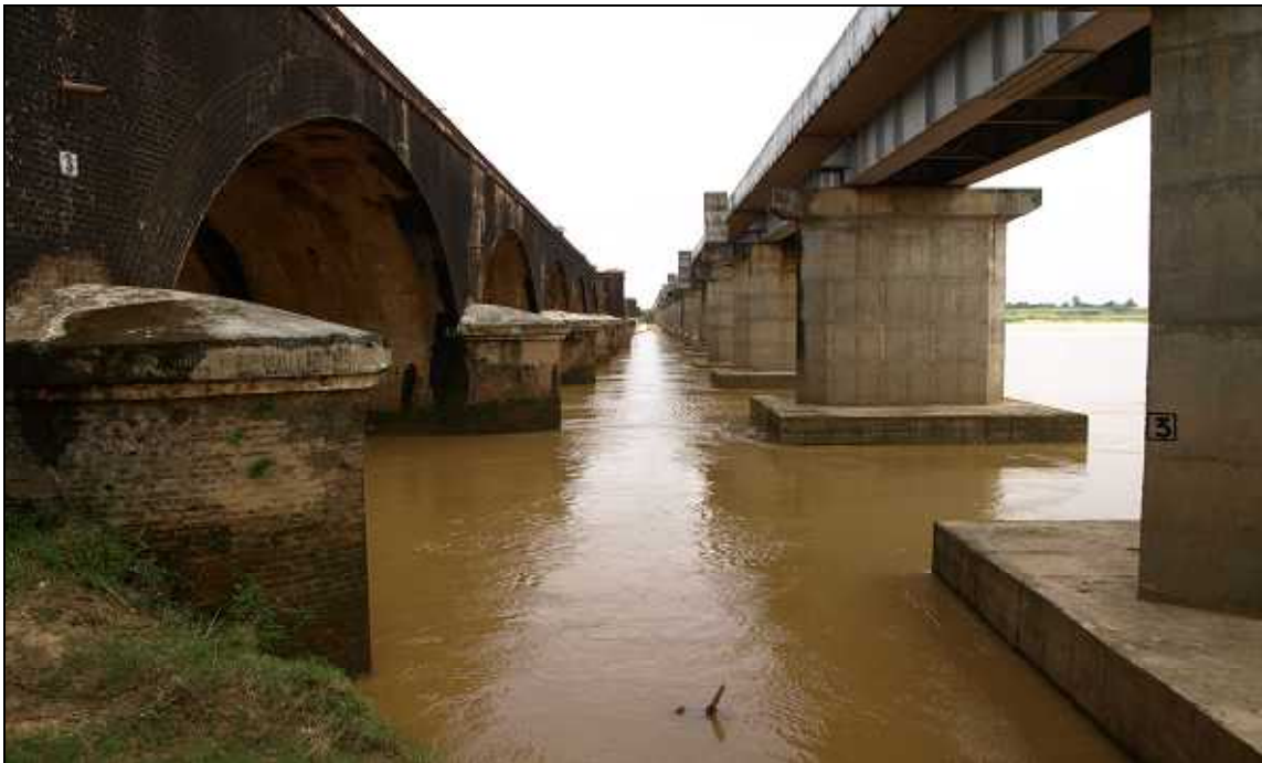
The old and new rail bridges side by side. The bridge on the left with arch shaped pillars is the old one.
