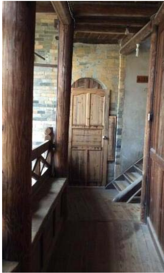
Figure 5.11 The blockage along a hallway
