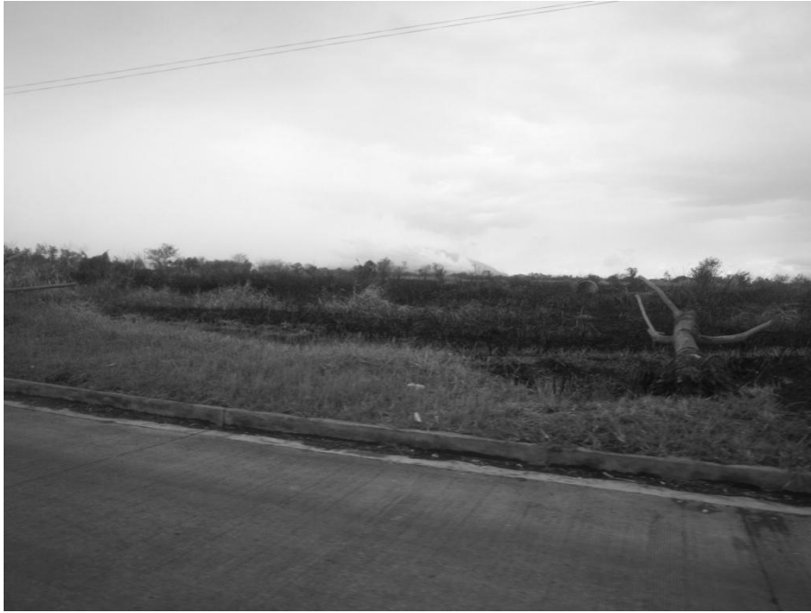
Figure 6.10: The lands are cleared by using fire, which sweeps through the grasslands in the dry season. A portion of the Nuvali land that is yet to be developed. (Photograph by the researcher March 12, 2010)
