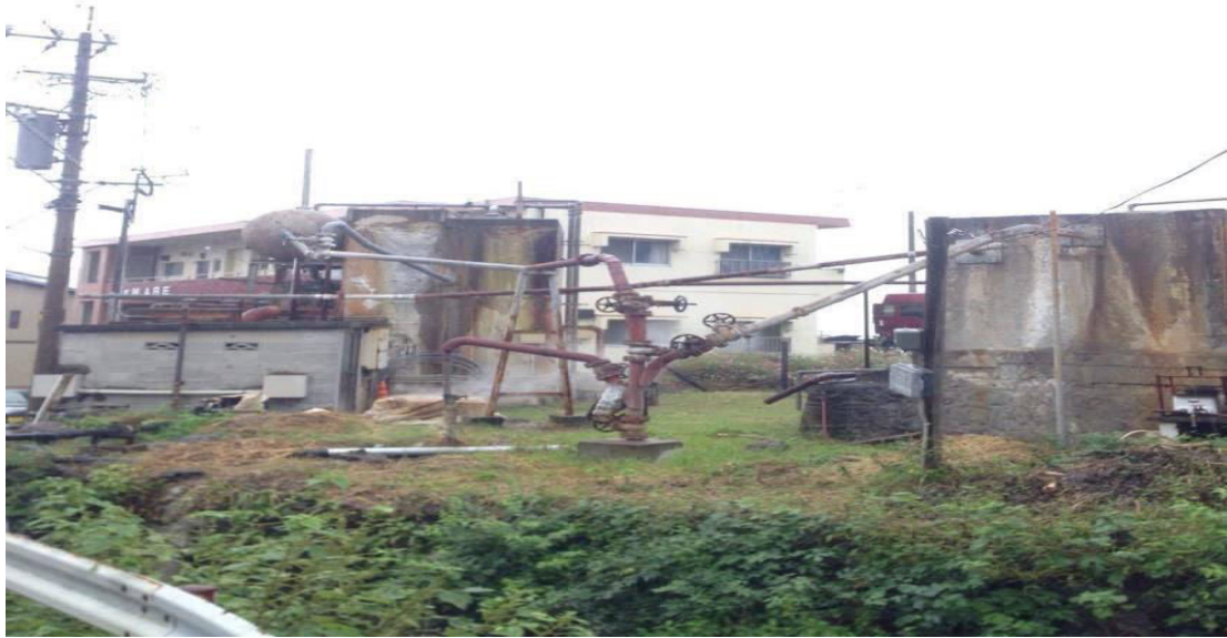
Image 2: Conventional hot spring extraction, cooling and distribution facility without binary hot spring geothermal generation unit in Kanawa district, Beppu city Source: Author
