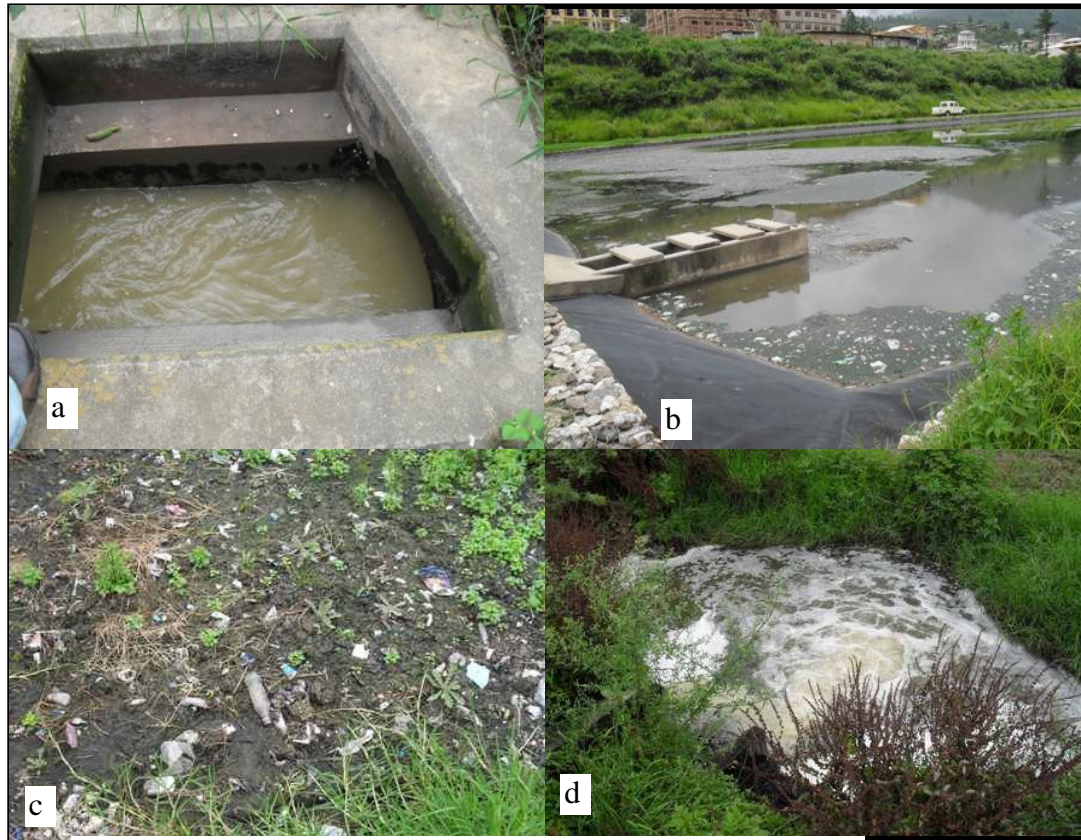
Figure 6. 3: Thimphu City's only sewage treatment plant (Lagoon); a- Inlet, b-treatment tanks, c-sludge, d-outlet/ treated water into river
