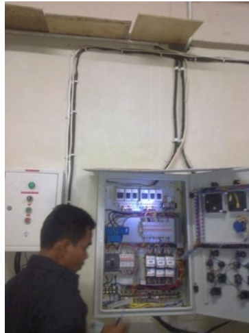
Picture 6.2. The leakage in panel room
