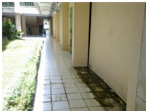
Picture 5.6. Leakage in ground tank (outside)
