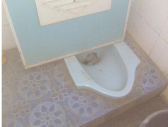
Picture 5.12. Condition of toilet after blown up
