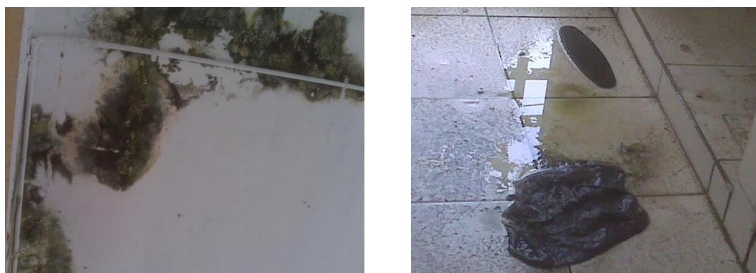
Picture 5.2. The leakage of dwelling unit
