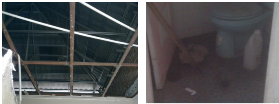
Picture 5.9. Damages in Rusunawa building
