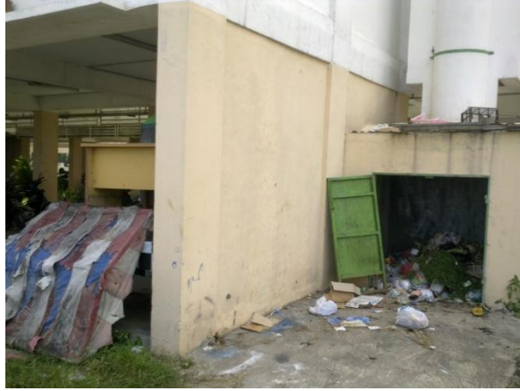
Picture 6.3. Condition of garbage shaft
