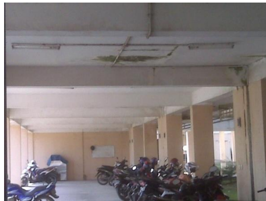
Picture 5.5. Leakage in parking area and hall
