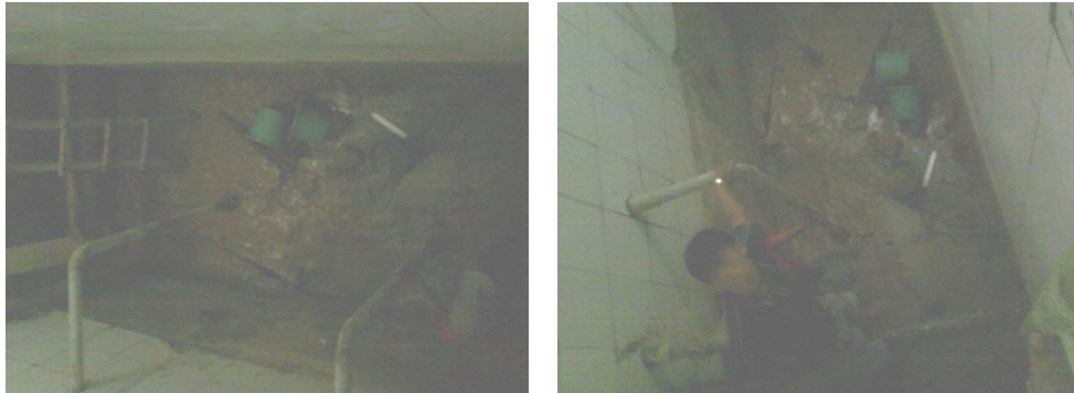
Picture 5.8. Dewatering ground tank
