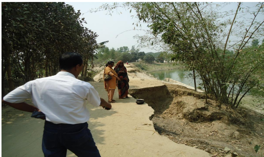
[Photo: The Main Pakka road at Bahuli Union, Destroyed by Flood and Inadequate Drainage System]
